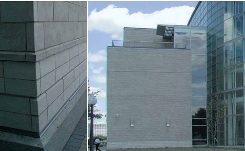
Masonry raised above grade
